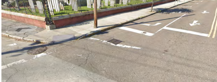
Existing pavement markings worn out
