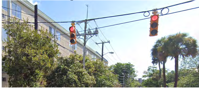
Existing Vanderhorst St. signal heads without retroreflective backplates.
