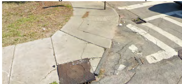
Sidewalk at Line St. approach needs to be repaired.
