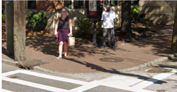
Sidewalk without detectable warning surface at Calhoun St.
