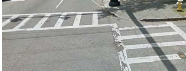
Existing pavement markings worn out
