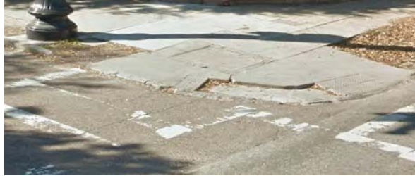
Sidewalk at Mary St approach needs to be repaired.
