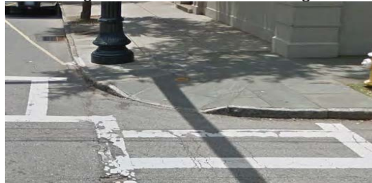
Sidewalk without detectable warning surface at John St.
